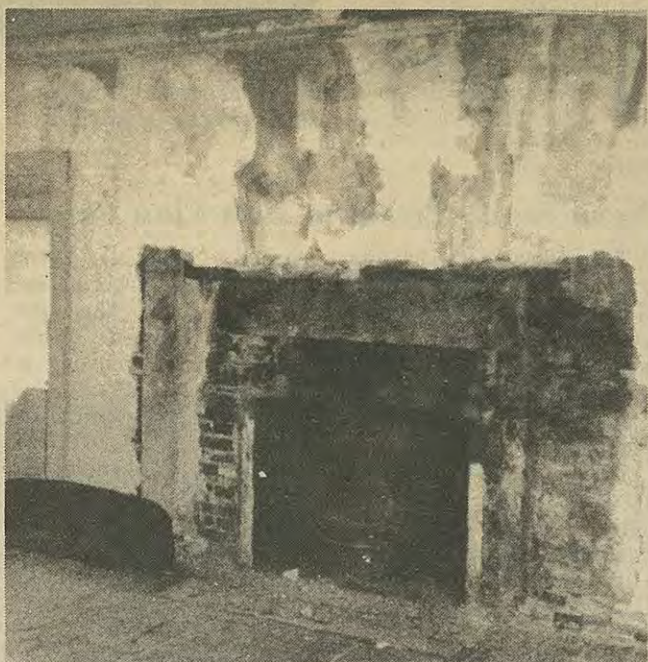
PILLAGED FIREPLACES in Castle Grant have ruined the historical aspect of most of the rooms, Mr. and Mrs. George Grant found on a visit in December. Most of this happened in the past two years.
